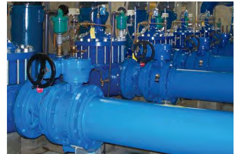
Graham Reservoir Pump Station
