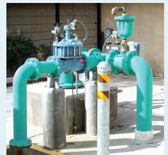
City groundwater supply well
