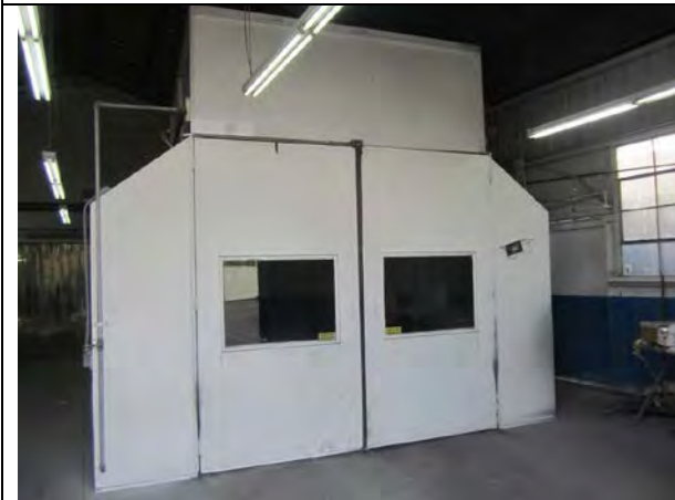
View of spray booth at A-Superior Collision Shop
