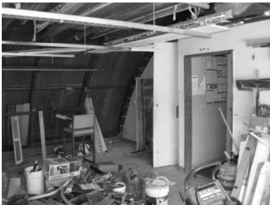
Photo 11. Another view of an unfinished interior area.
